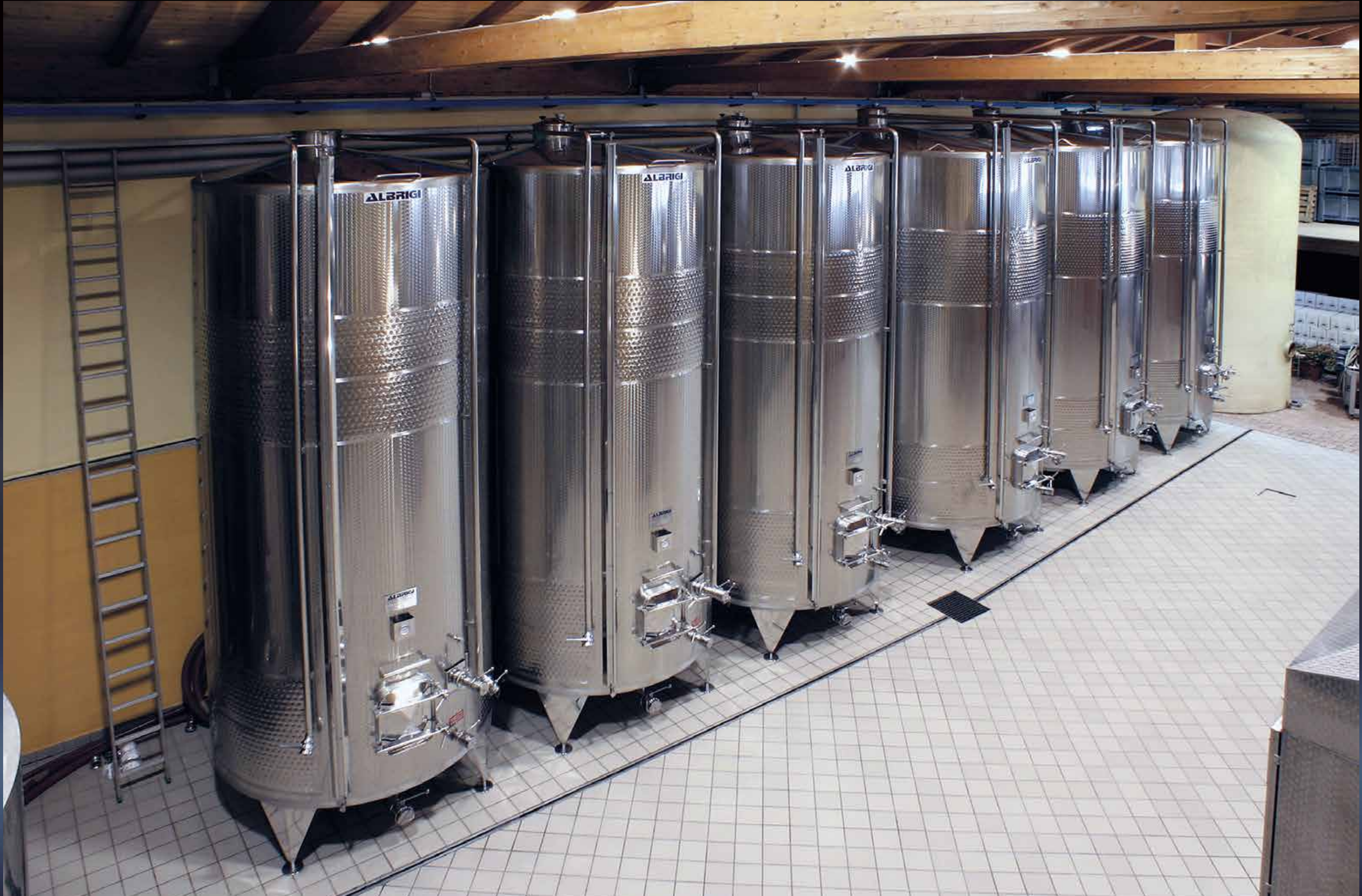
150 hl Vinotank, temperature controlled by Termostar Double and fitted with Cleanfix washing plant
