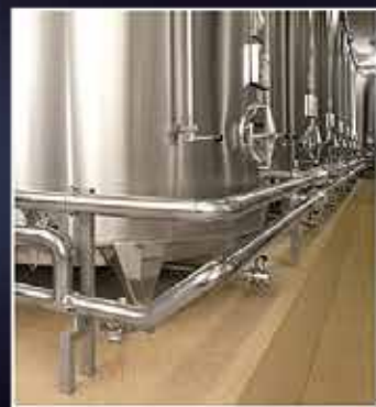
Stainless steel piping
