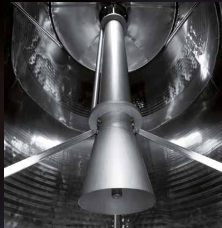
Turbotank "Termo", patented by Albrigi, installed inside a 600 hl fermentation tank
