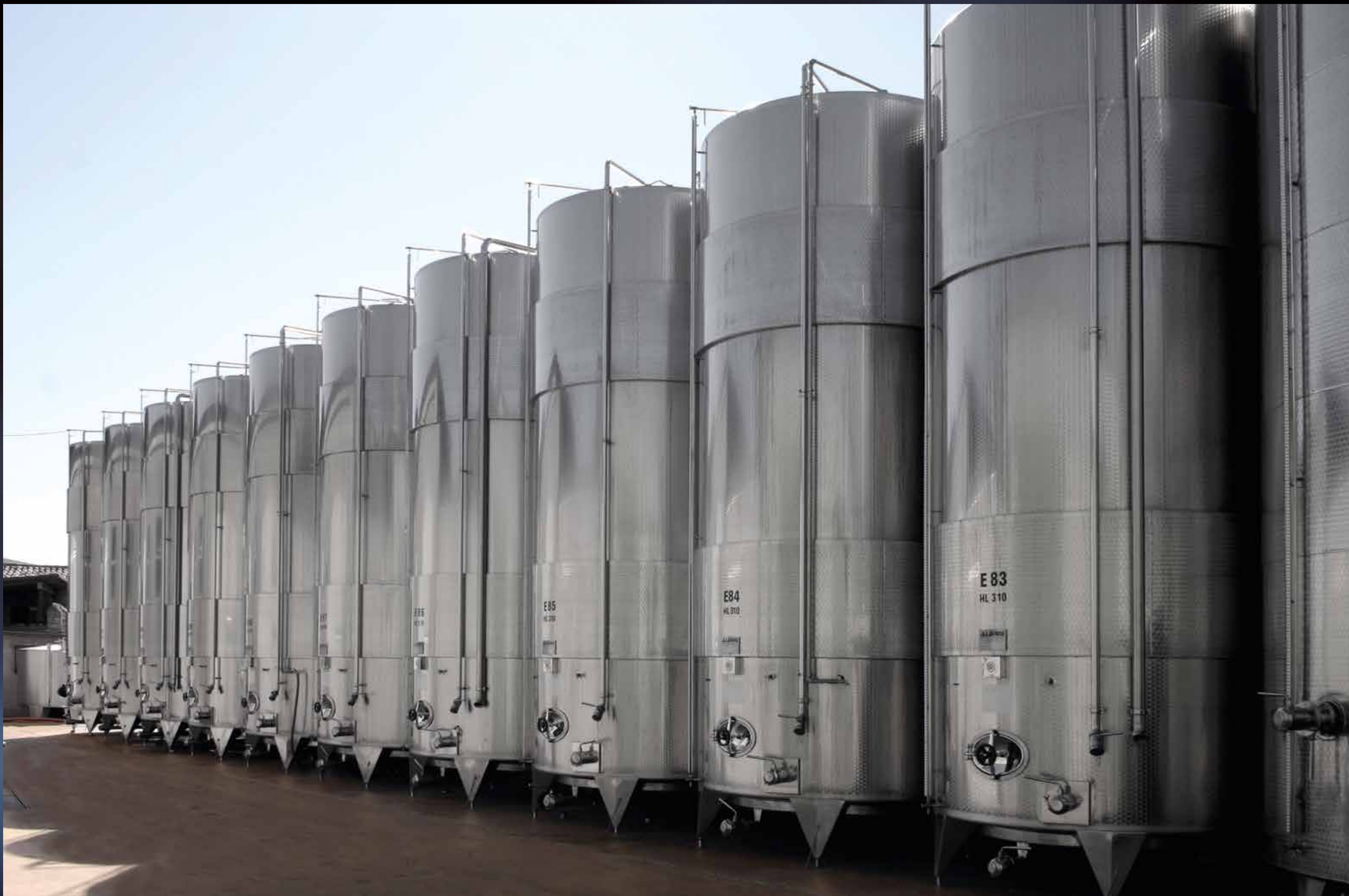
Bank of Termotank Double Tanks, temperature controlled by Termostar, fitted with Isoplus on the jacket & Cleanfix washing plant
