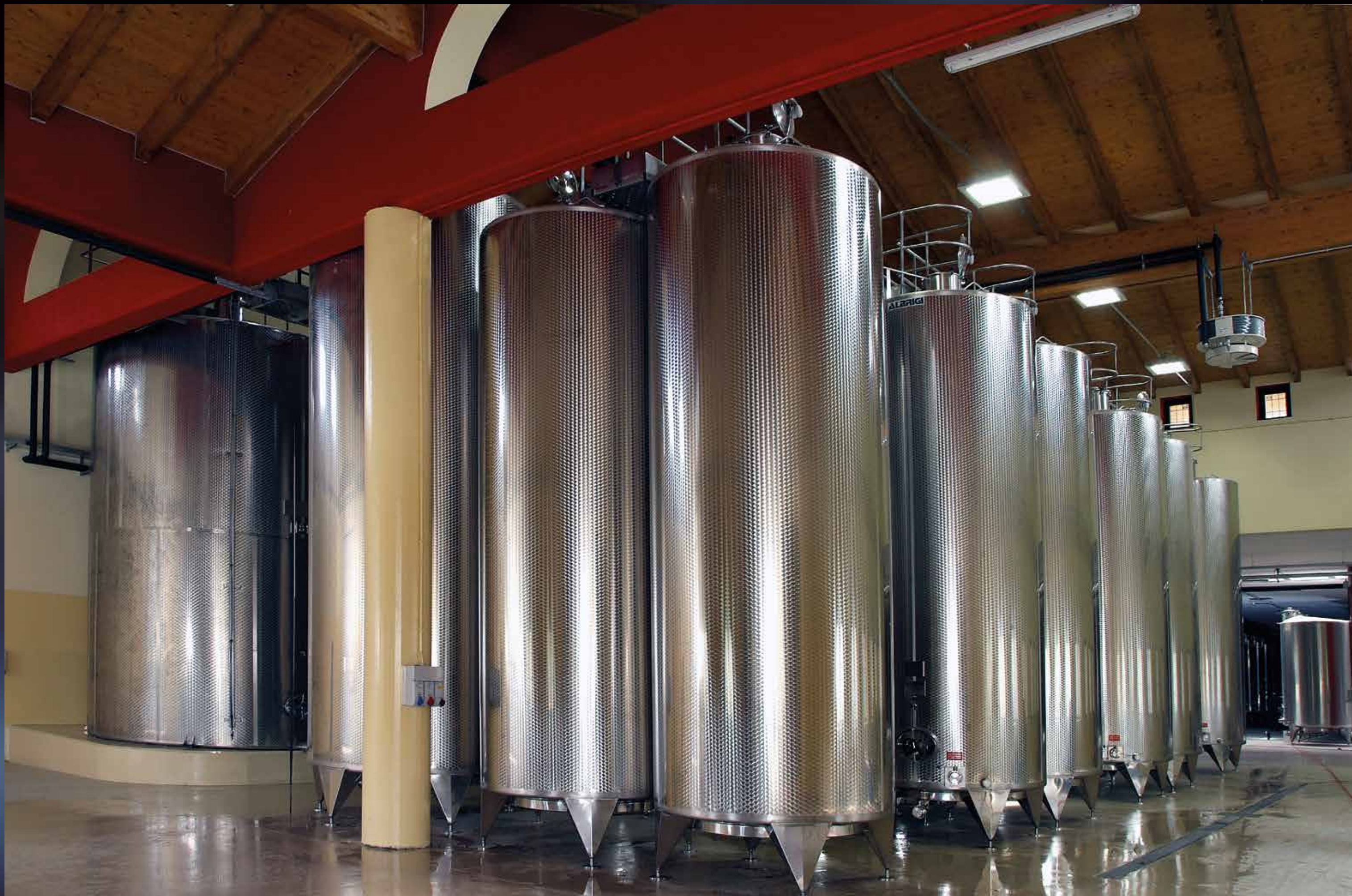
150 and 600 hl Vinotanks with service gangways and landing accessing every manhole cover
