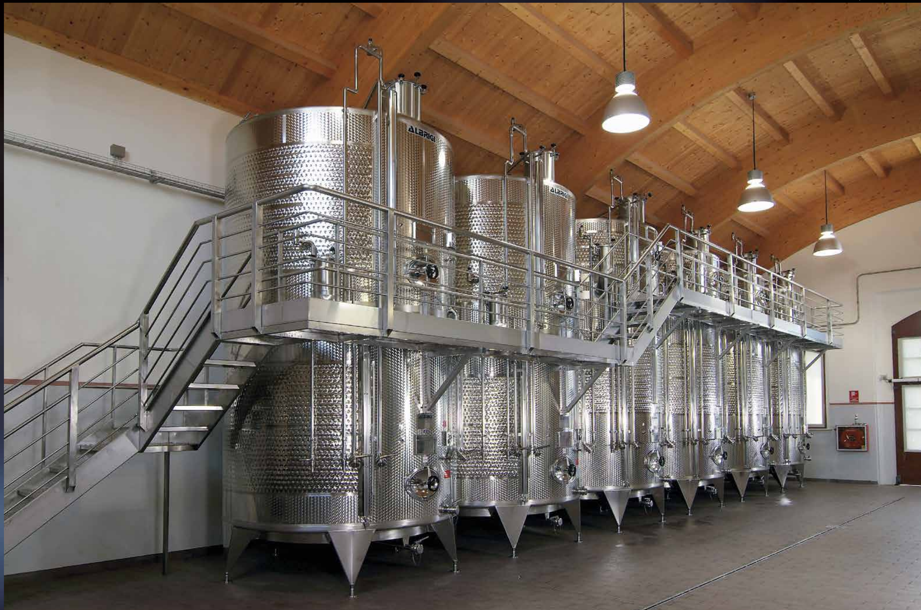
100 + 100 hl Politanke Termo Tanks, temperature controlled by Termostar, fitted with Cleanfix washing plant and Innergas
