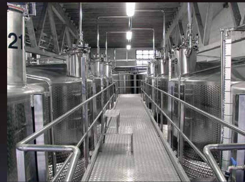
Gangway with 300 hl tanks, safety unit and "Innerpipe" system of fixed stainless steel pipes
