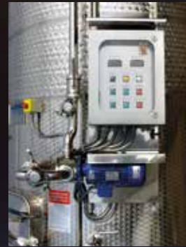
Electric board controlling the pump over pump or the punching down phases
