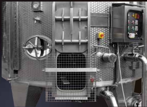
Guillotine door with protective cage
