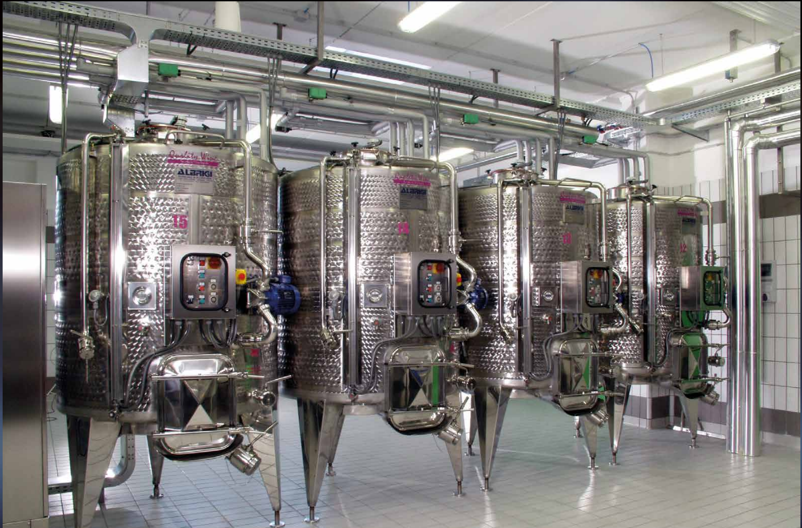
25 & 20 hl Specialtank winemaking tanks, temperature controlled by Termostar, fitted with delestage and pump-over pump
