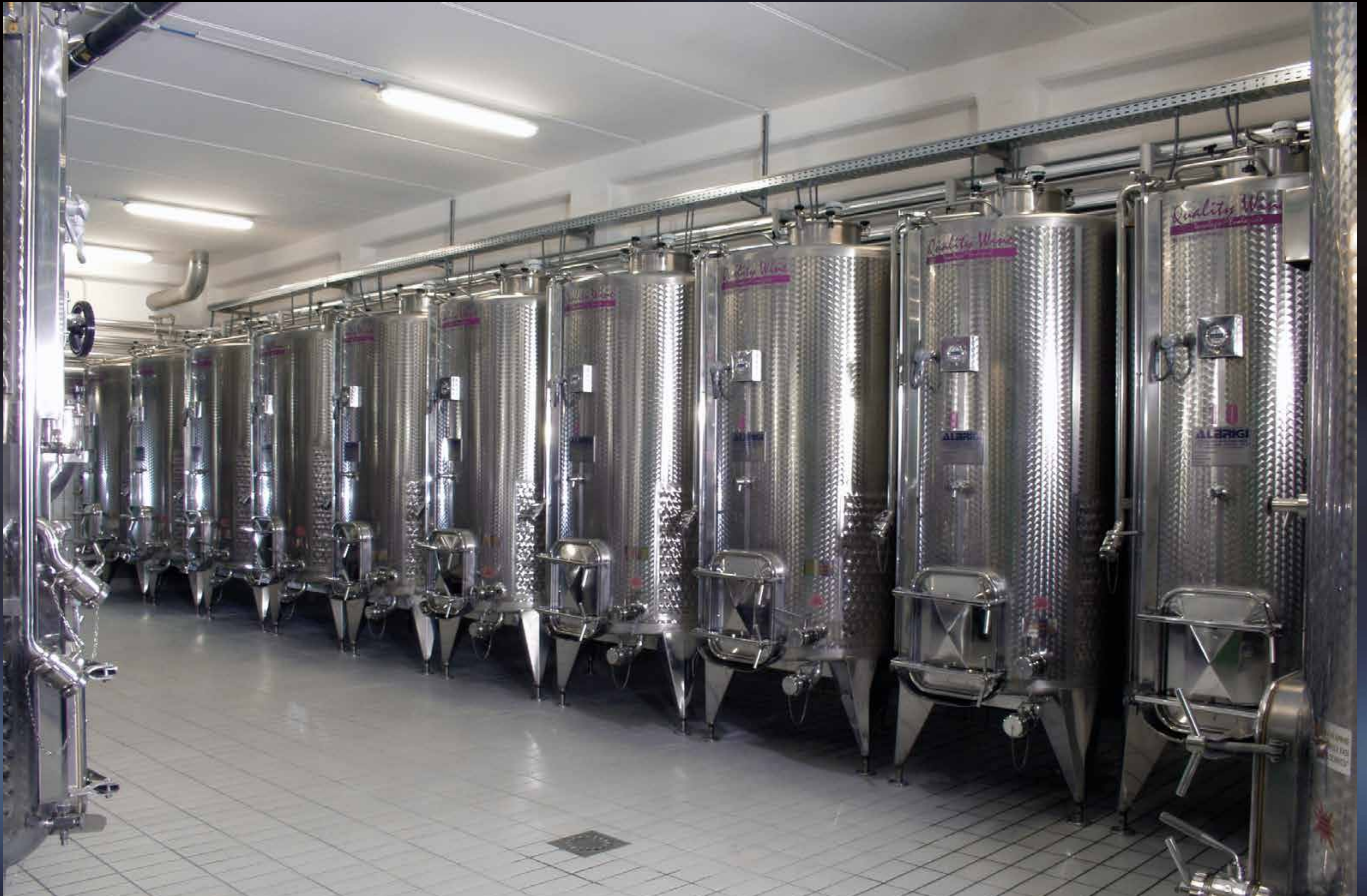
Specialtanks, temperature controlled by Termostar and fitted with fermentation accessories
