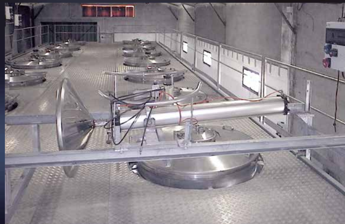
Punching down mechanism on a double rail overhead traveling beam with the single foot in its at-rest position
