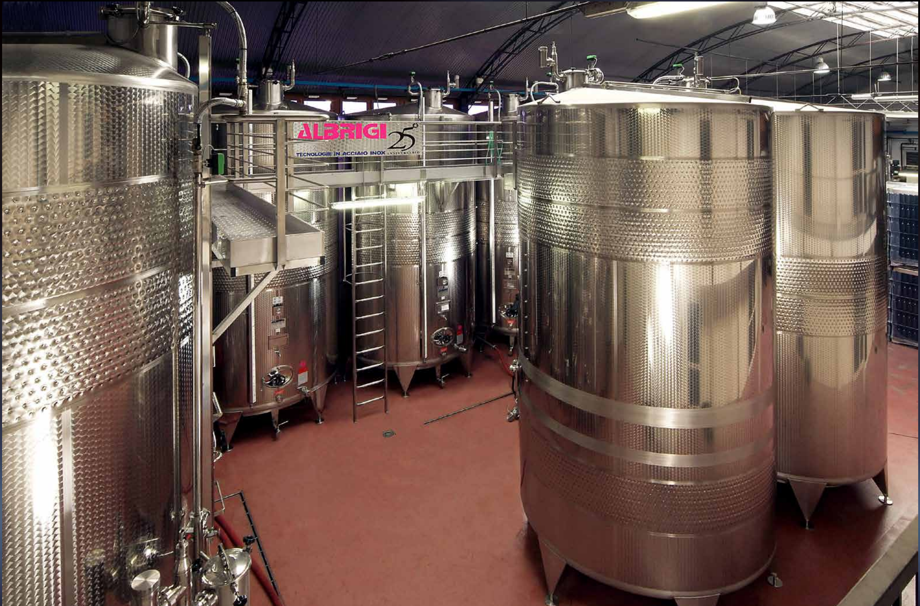
300 hl Termotank, 150 + 150 and 200 hl + 100 hl Politank Thermo tanks all with Innergas, Cleanfix washing plant and service gangways
