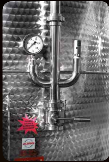
Safety unit with PED calibrated safety valve and pressure gauge
