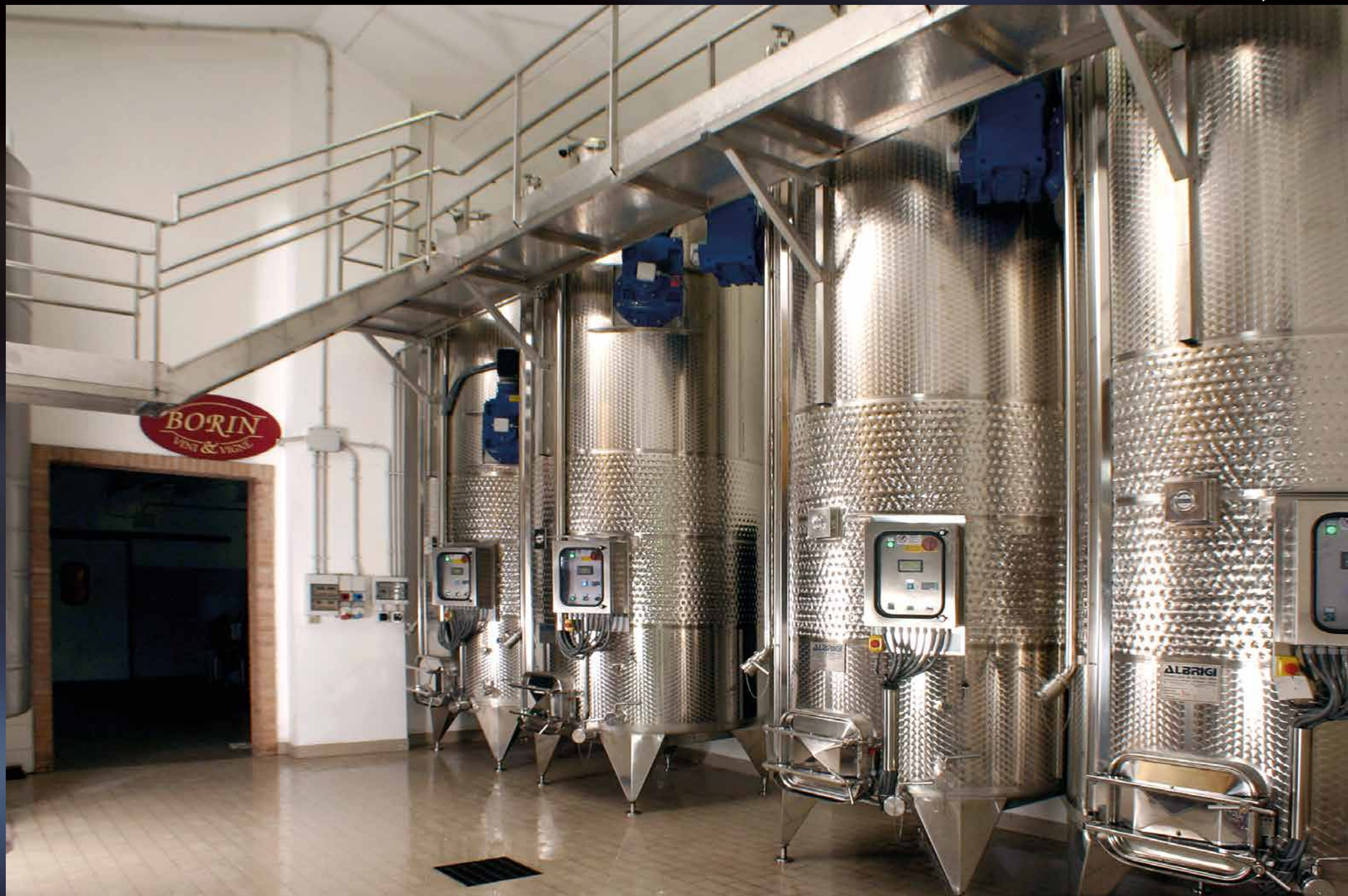
Wine Cellar with 100 hl Volvotank, temperature controlled by Termostar and fitted with Cleanfix washing plant
