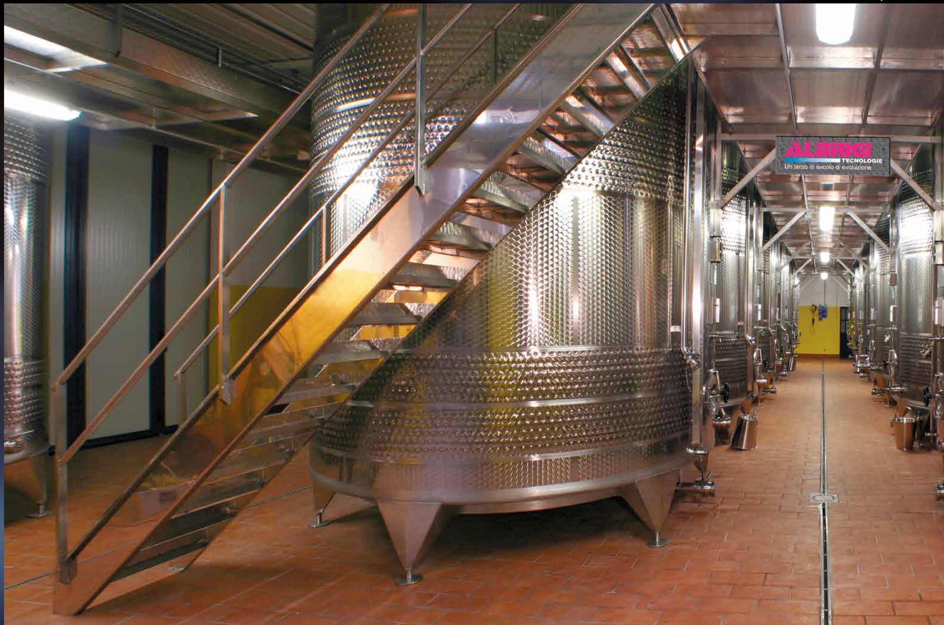
Fermentation Cellar with 300 hl Termostar tank; temperature controlled by Termostar Double and fitted with Cleanfix washing plant
