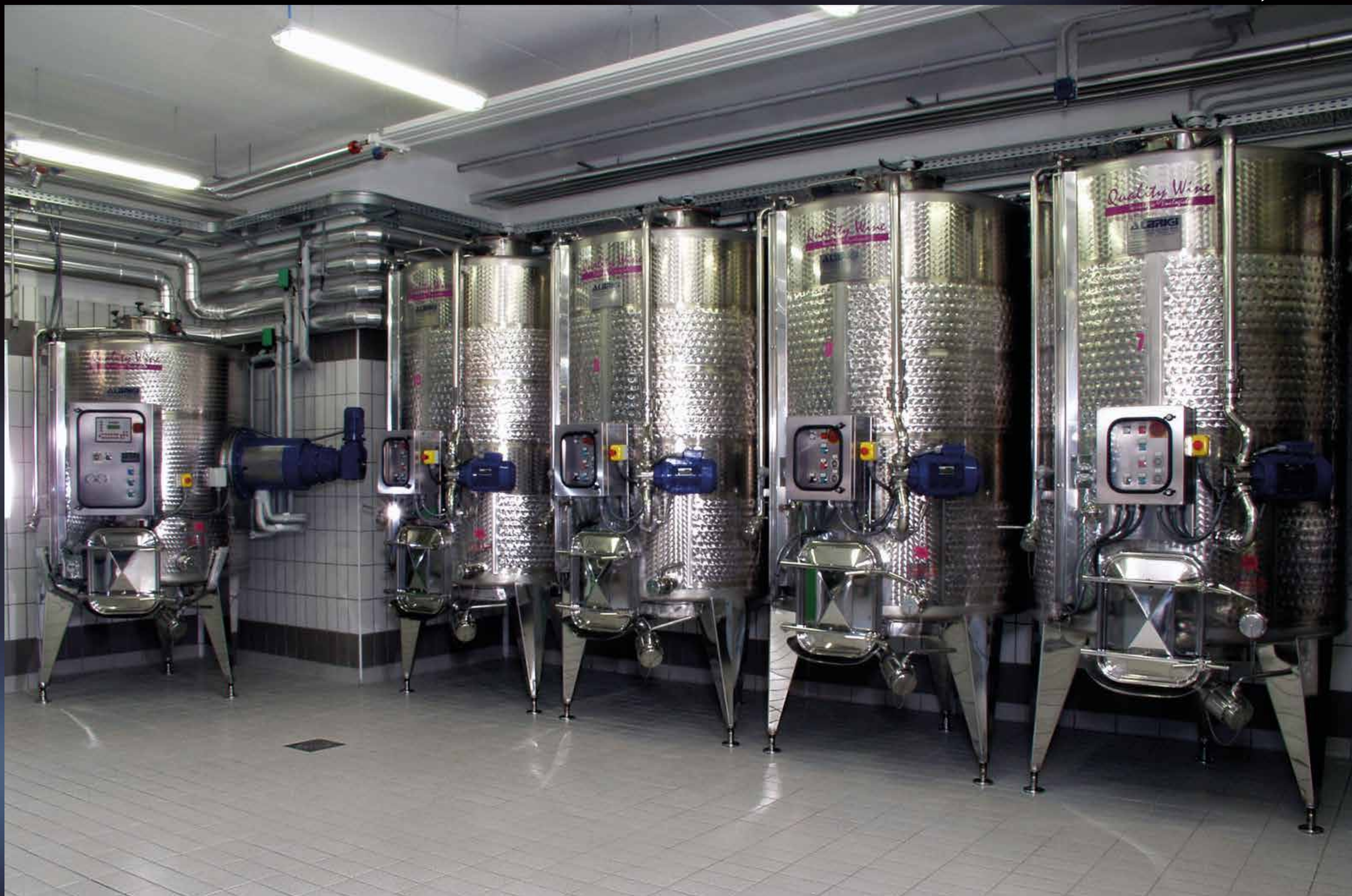
20 hl Volvotank & 25 hl Specialtank fermentation tanks temperature controlled by Termostar and fitted with pump-over pump
