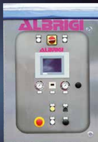
Stainless steel electric board with protective PVC rolled up curtain and PLC that programs all pause/work phases
