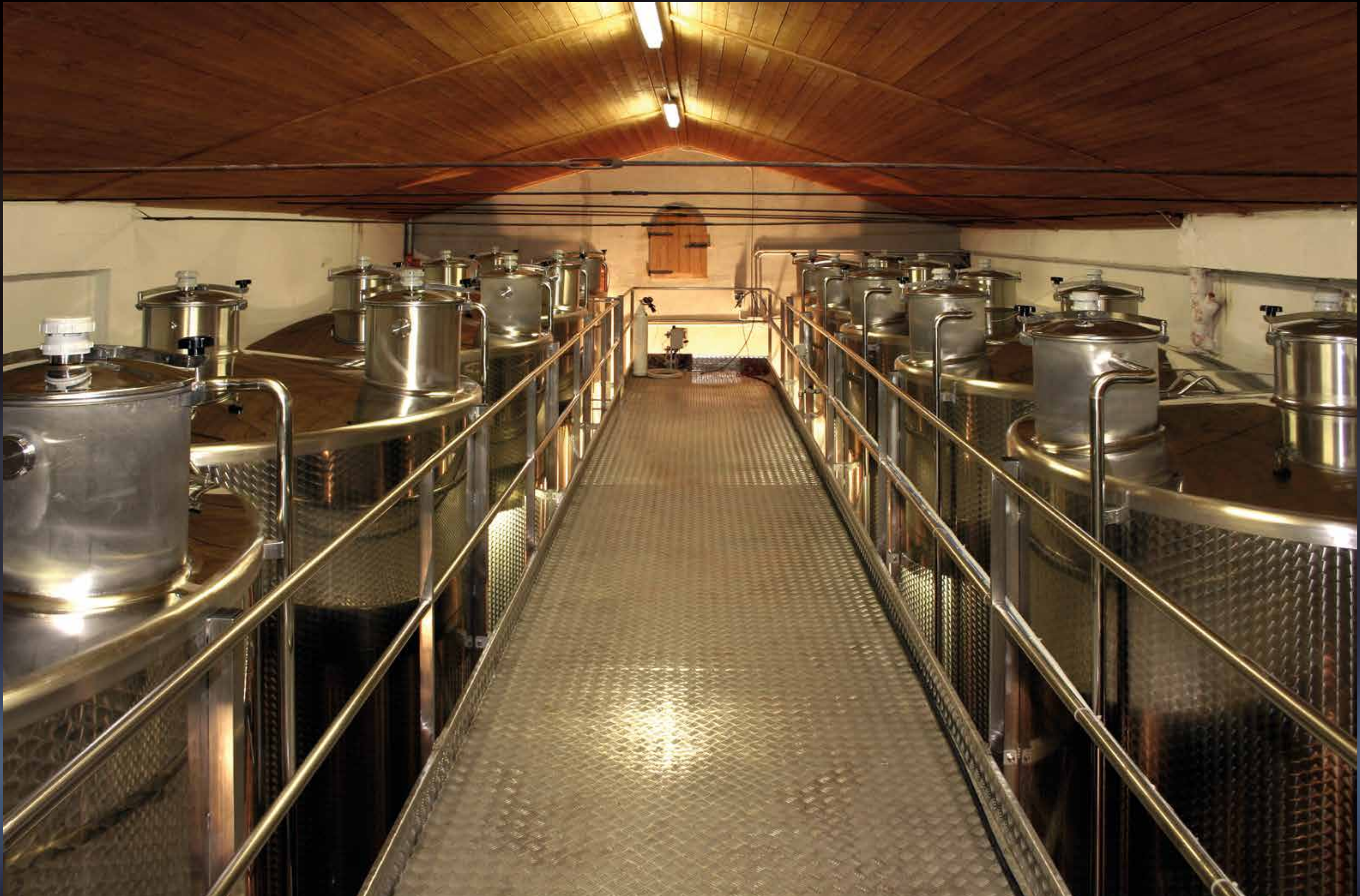
Specialtank 200 hl fermentation cellar
