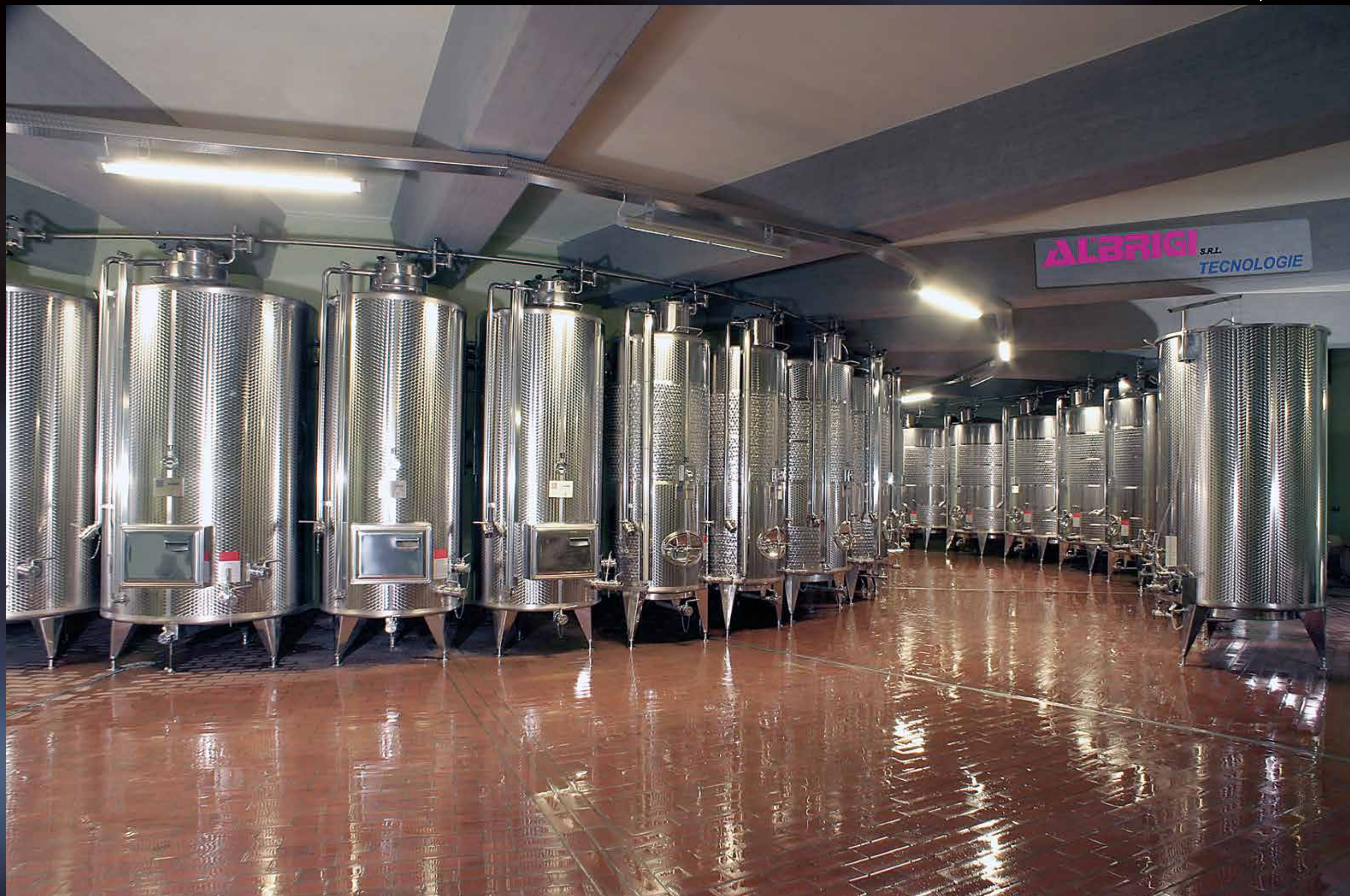
Wine Cellar with 50 and 25 hl Frigotank, and hl 100 and 50 hl Termotank
