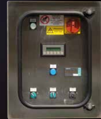
Board for automatic temperature and stirrer control
