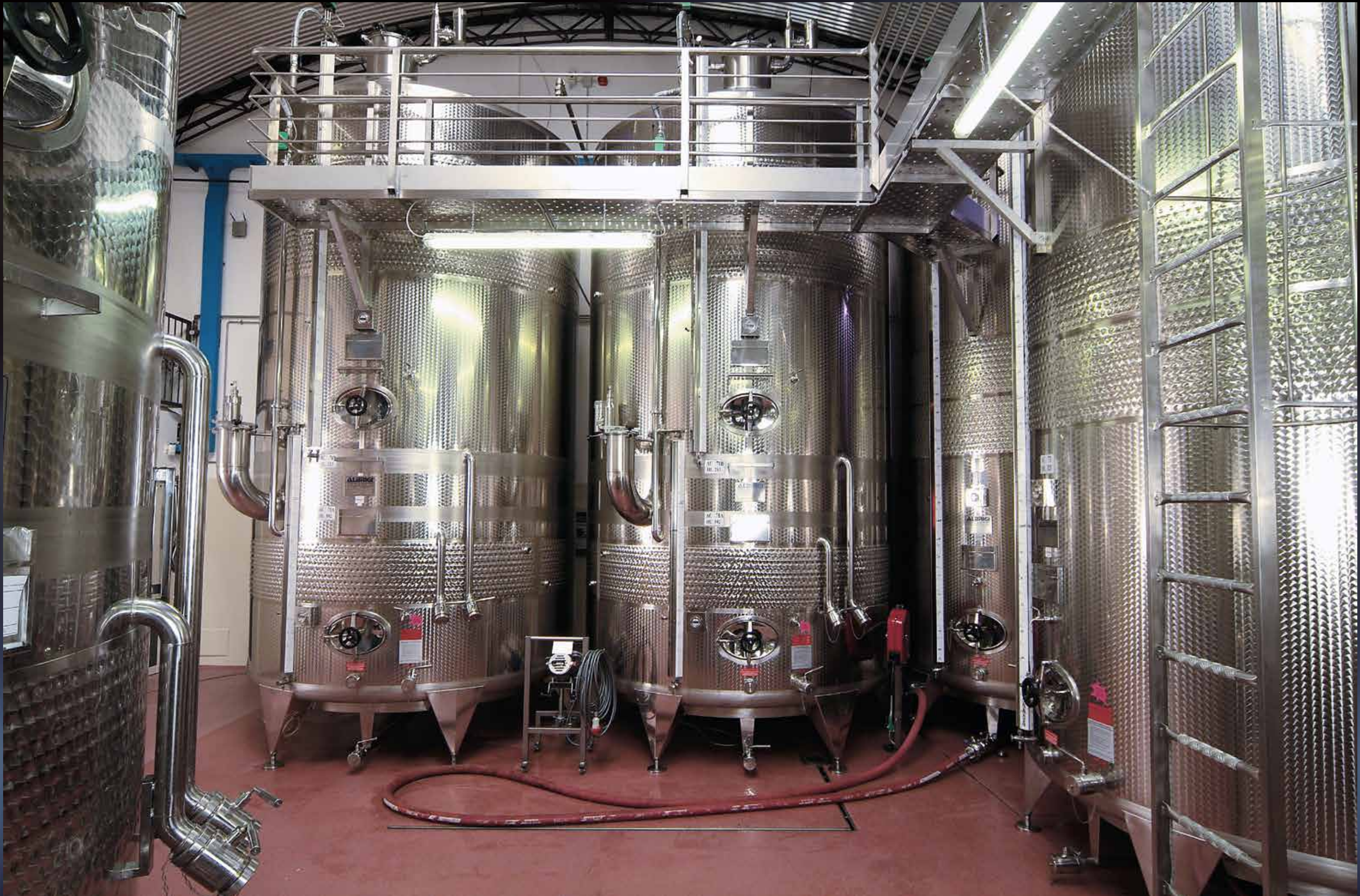
100 + 200 hl Politank Termo Tanks and 200 hl Termo Tank, temperature controlled by Termostar, fitted with Cleanfix washing plant and Innergas
