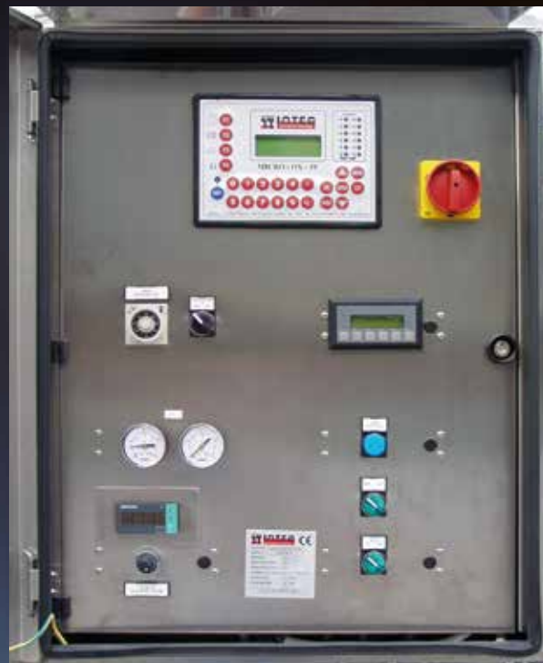
Board with oxygenation control unit
