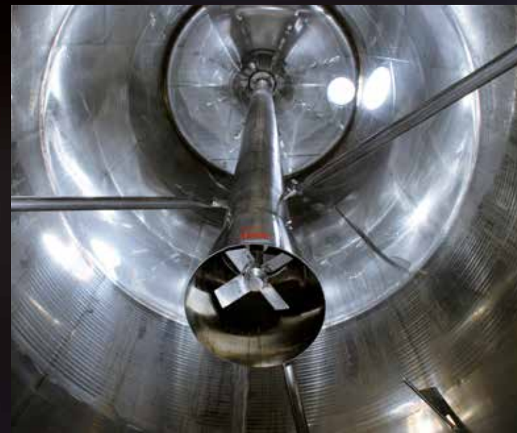
Turbotank installed inside a 1000 hl fermentation tank
