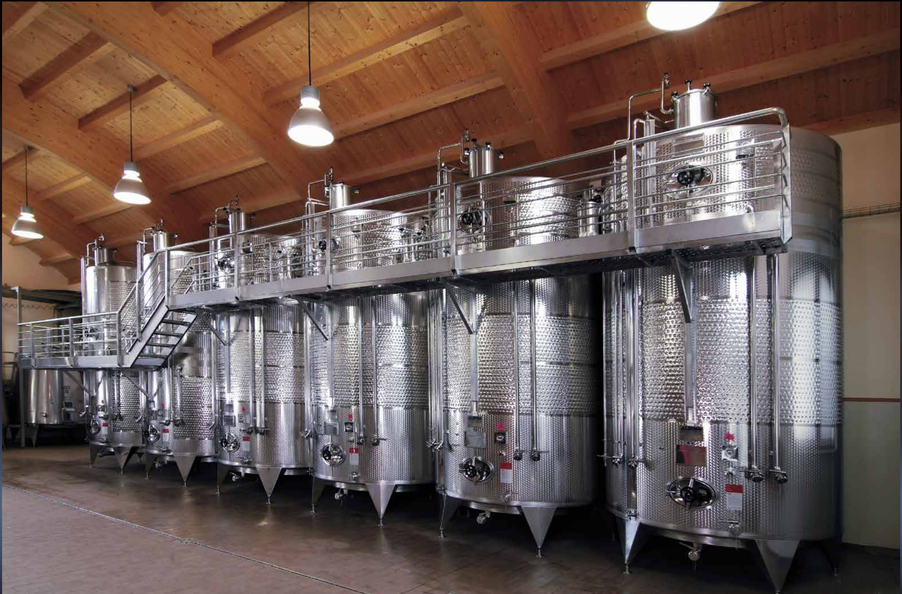
150 + 50 hl Politank Thermo Tanks, temperature controlled by Termostar, fitted with Cleanfix washing plant and Innergas
