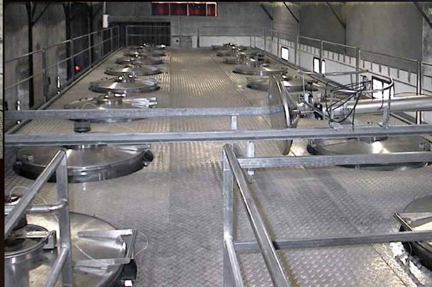
View of Superfollrail with twenty 200 hl fermentation tanks and the single punching down foot in its at-rest position
