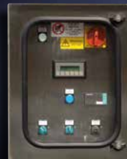
Control board for temperature and automatic pump over
