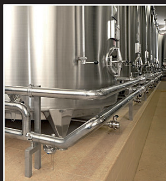
Inox connection pipes
